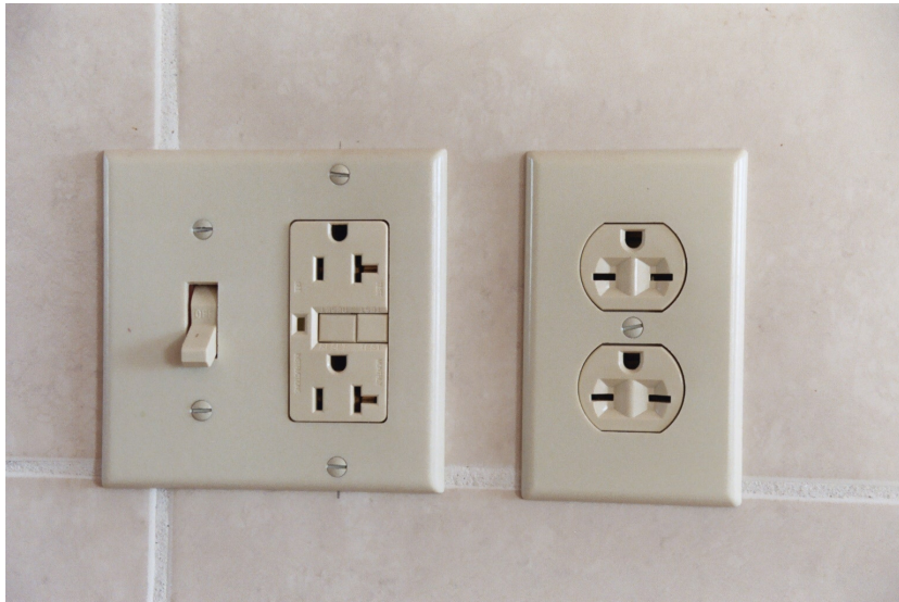
Switched GFCI outlet in kitchen. The right outlet is for DC electricity (see separate article).
