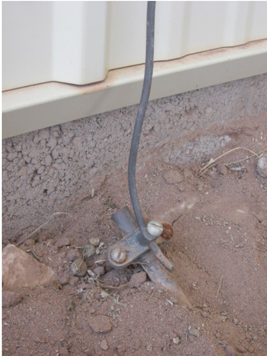
The ground rod is usually located right below the main electrical panel, with a wire connecting the two.
