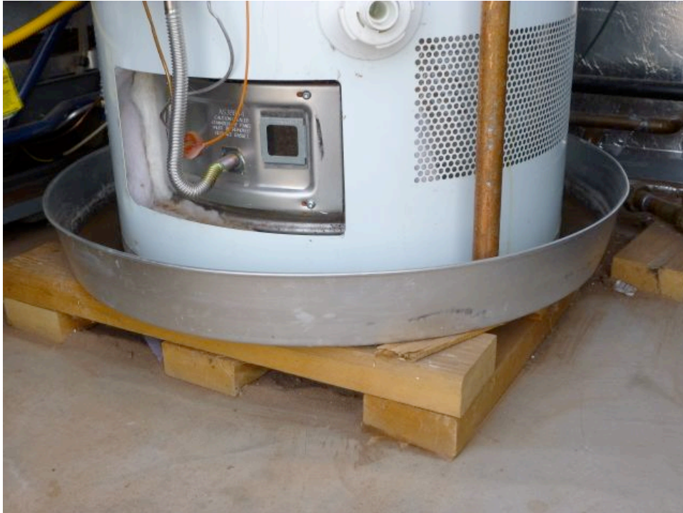
Gas water heater with a water-collection pan underneath.
