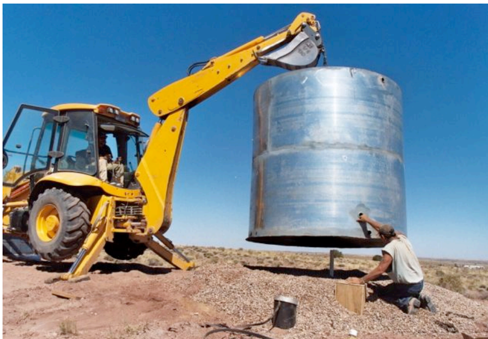
Installing a steel water tank on a gravel bed to prevent rust. The intake/outlet is in the bottom, to prevent freezing.
