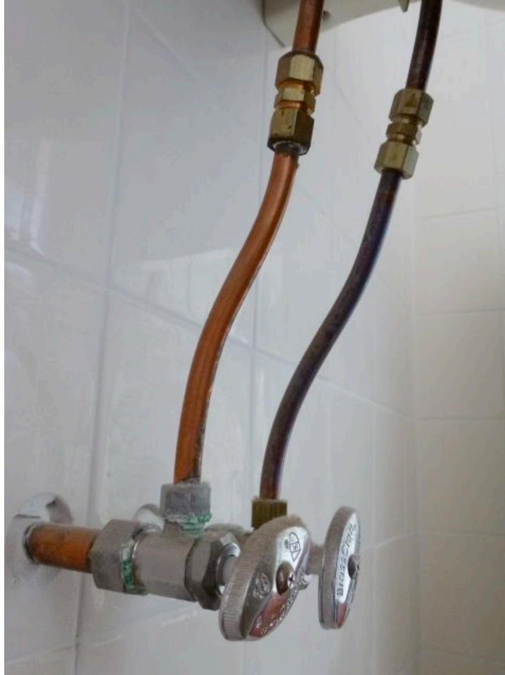
Flexible copper pipes used to connect a faucet.
