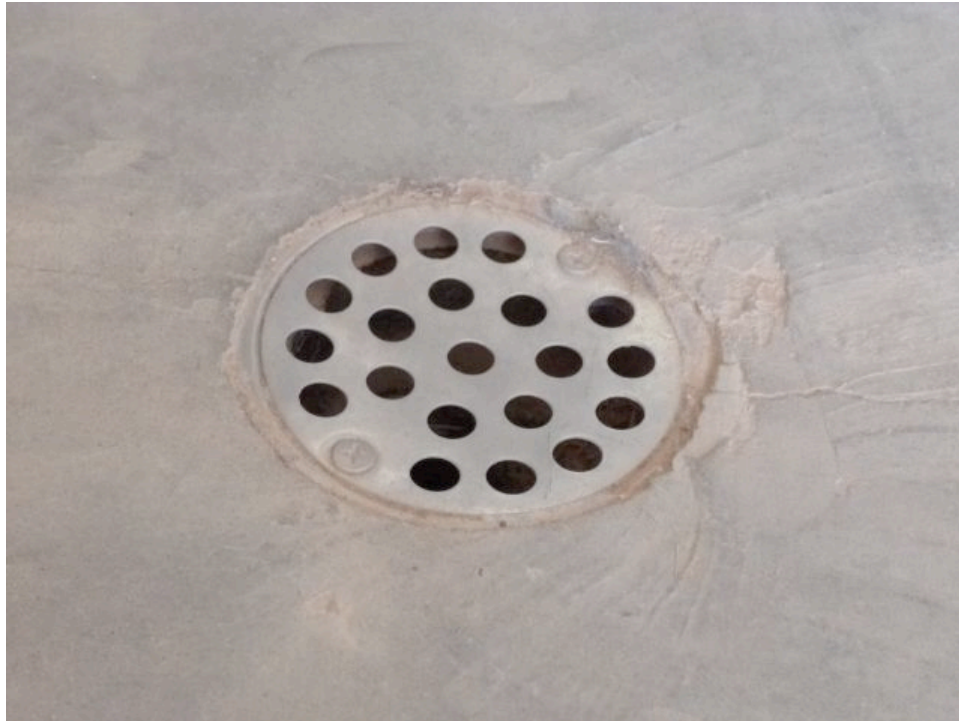
Floor drain in utility room protects against flooding
