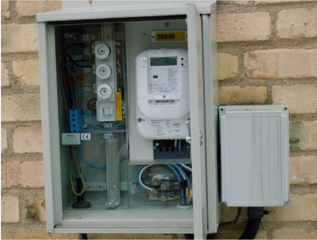
The E.ON filter is the box mounted on the wall to the right of the Lindblom family’s electrical meter.
