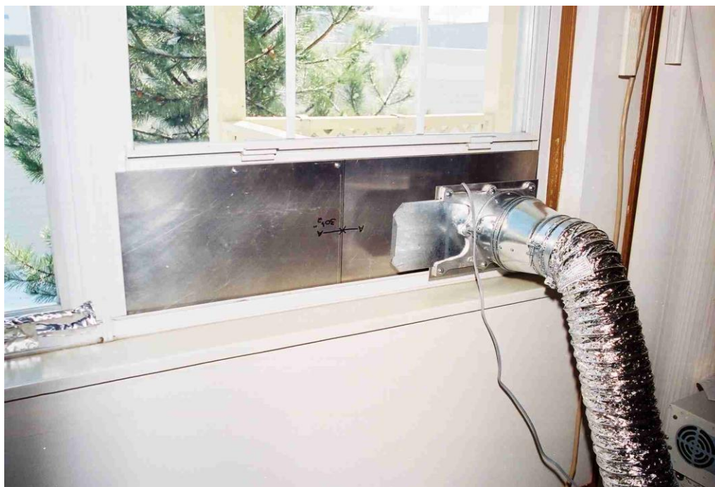
Suction fan exhausting fumes out through a window.
