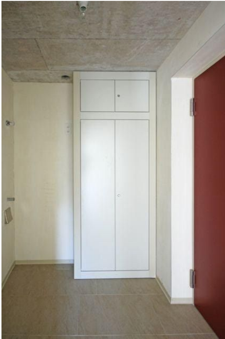
Airlock with utility closet, entrance door and air vent in ceiling. The washing machine has not yet been installed.
