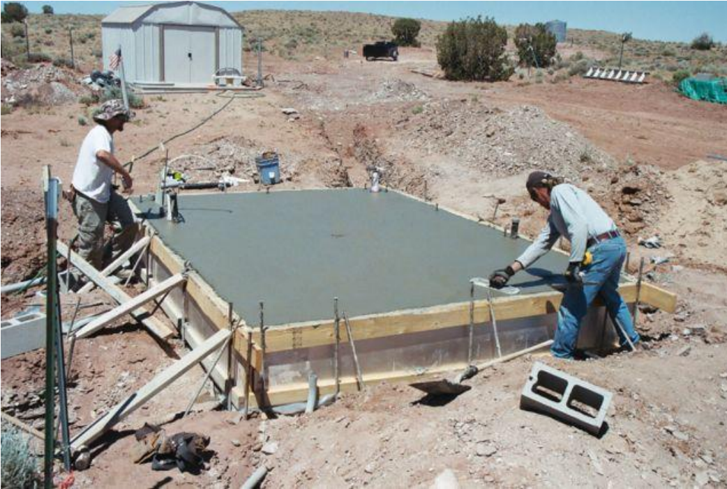
Insulated monopour foundation for a small outbuilding.
