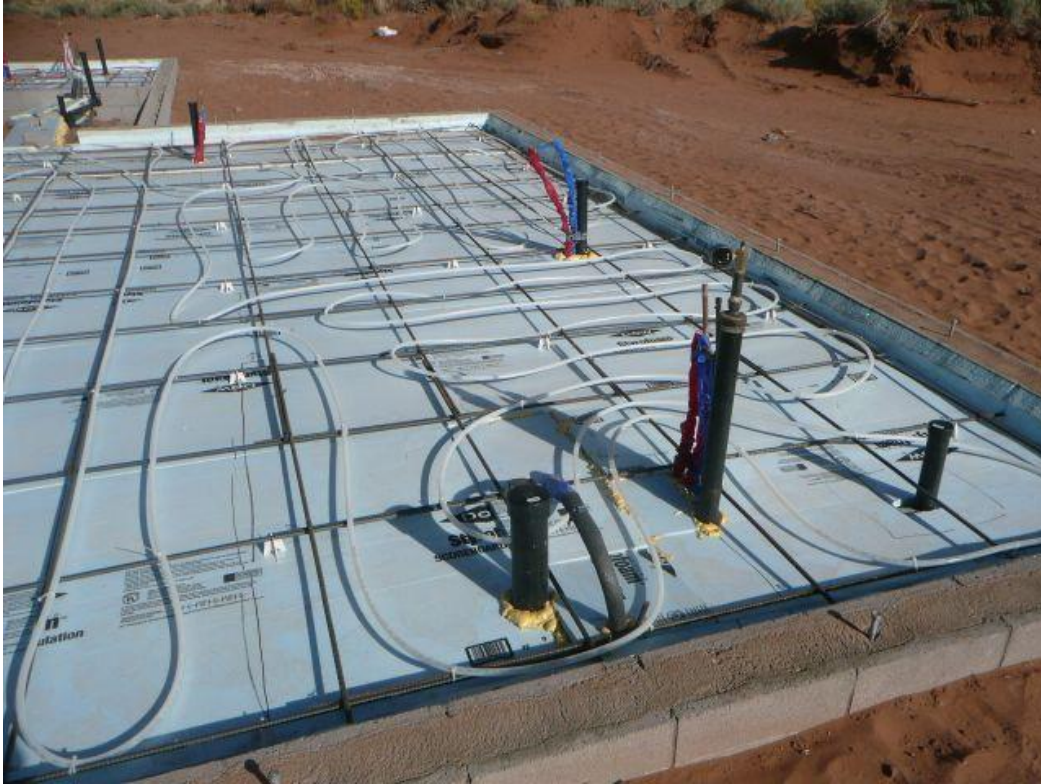
Foundation with radiant floor heating system, ready to pour the concrete slab.
