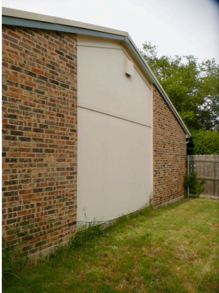
The exterior is mostly brick, which never needs painting. The wood panels at the end were replaced with cement siding.
