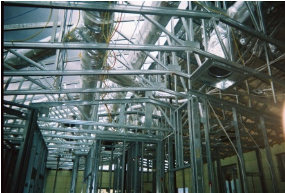
Rigid steel air ducts.
