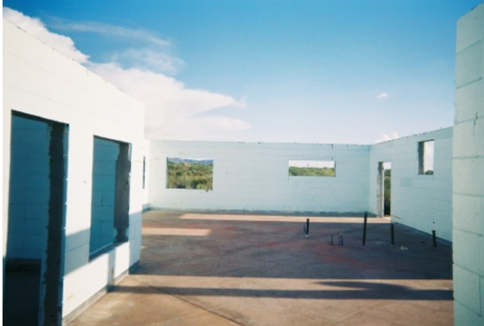
The polystyrene Integrated Concrete Forms create strong airtight outer walls. The floor is tinted and buffed concrete.
