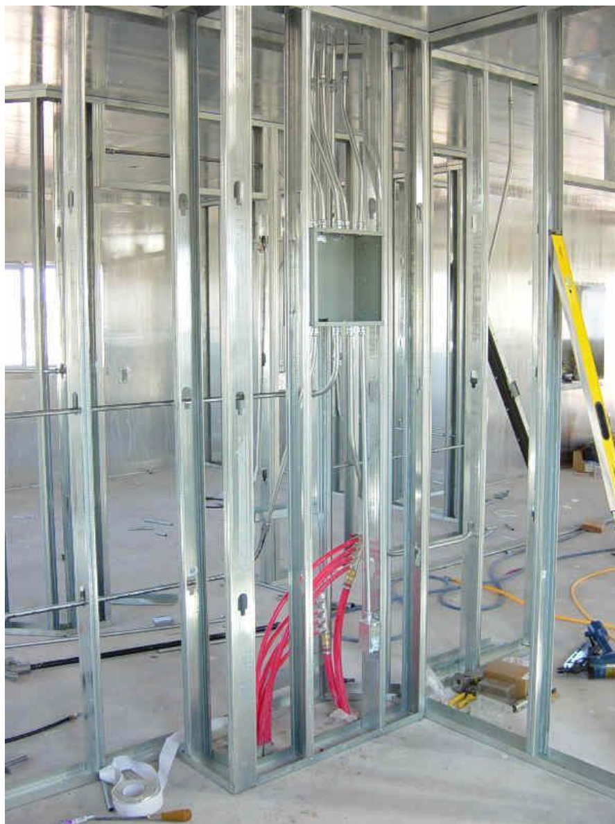
Steel studs can carry stray electricity.
