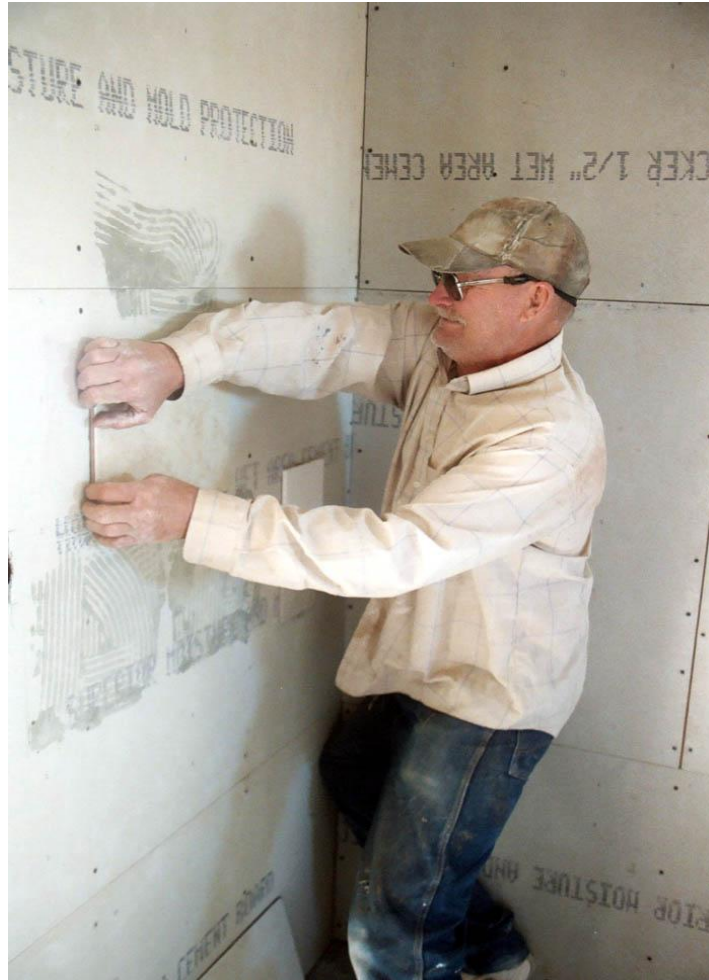
A tile worker testing the additive-free thinset recipe with a wall tile in the bathroom. The tile had to be chiseled off.
