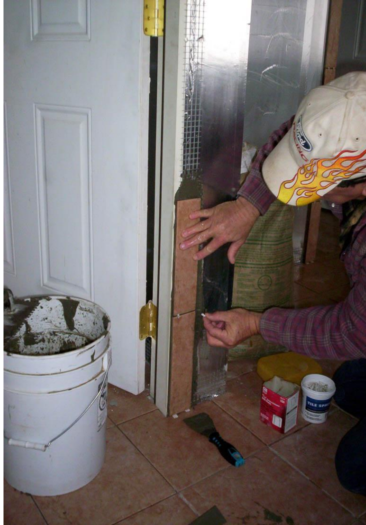
Setting the tile around door and baseboard, using steel mesh (1/2 inch hardware cloth) for extra strength in these areas. The drywall is sealed with an aluminum foil that is attached with wallpaper wheat paste.
