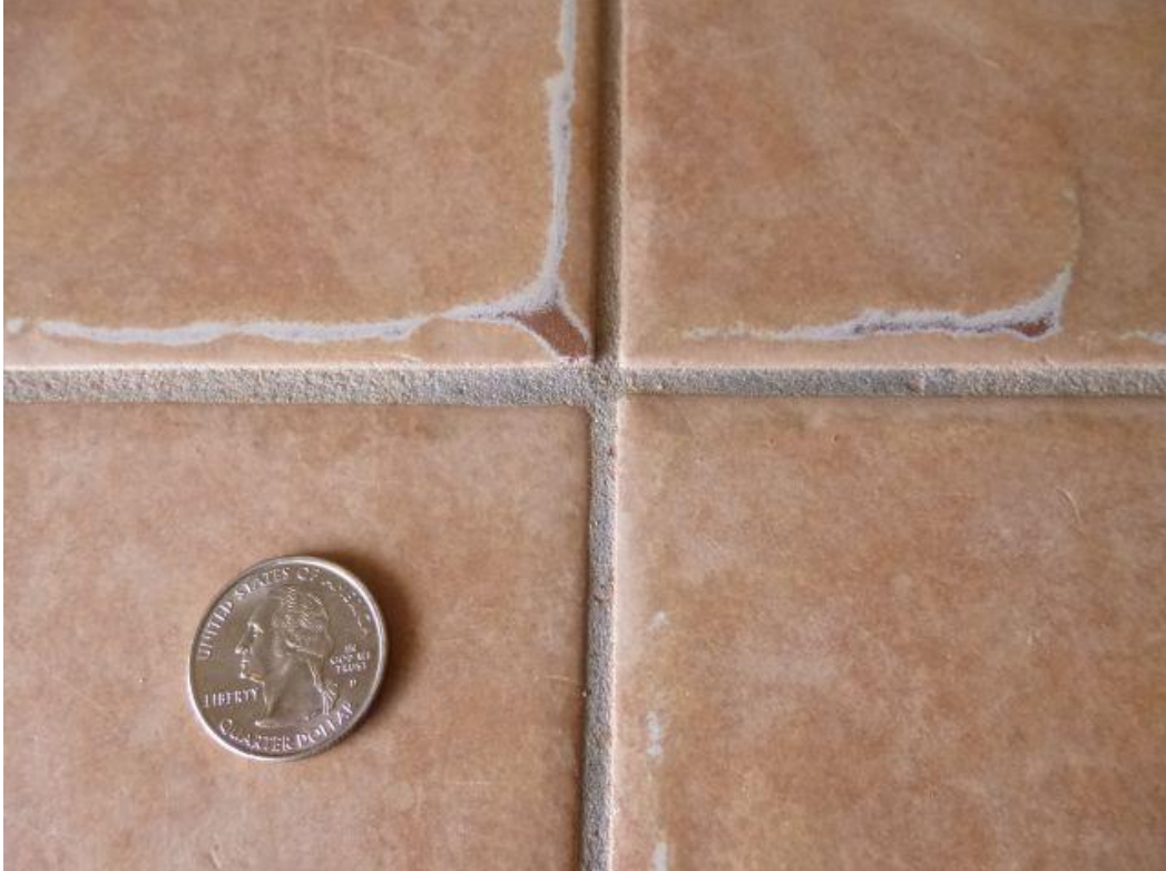
The edges of these low-cost floor tiles are starting to wear after six years in a high-traffic area.
