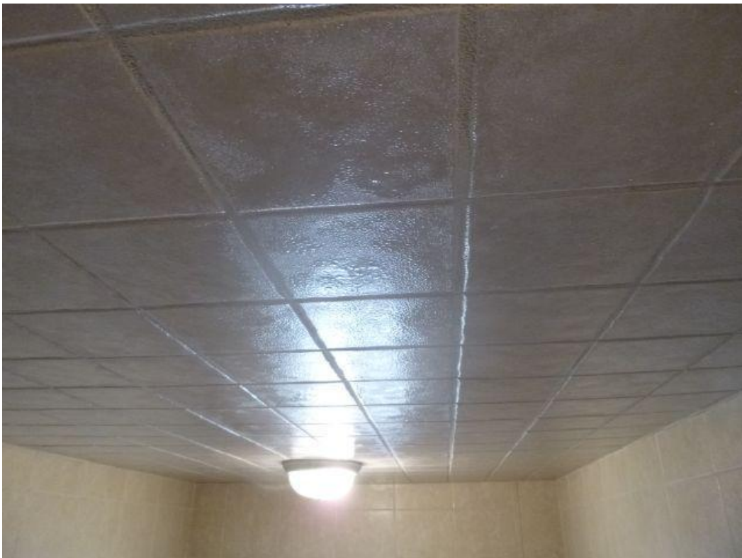
Wet ceiling after a shower, despite thick insulation (R-60) above the tiles.
