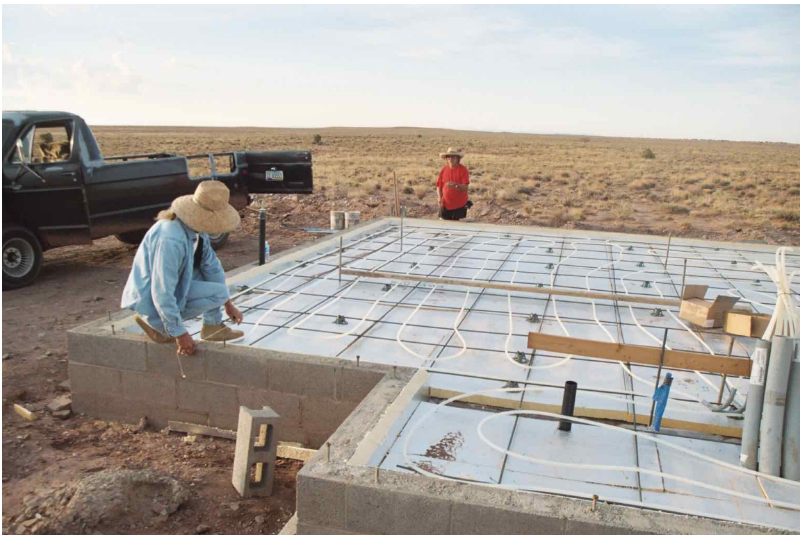
The concrete slab is ready to be poured. The PEX pipes and insulation can be seen.
