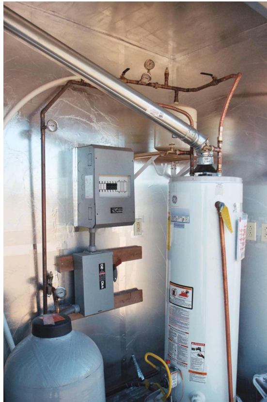
The gas water heater in its sealed-off closet, before the pipes were insulated.
