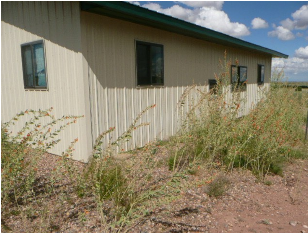
The outside of House-3, with steel siding, steel roof and metal-coated low-E windows.
